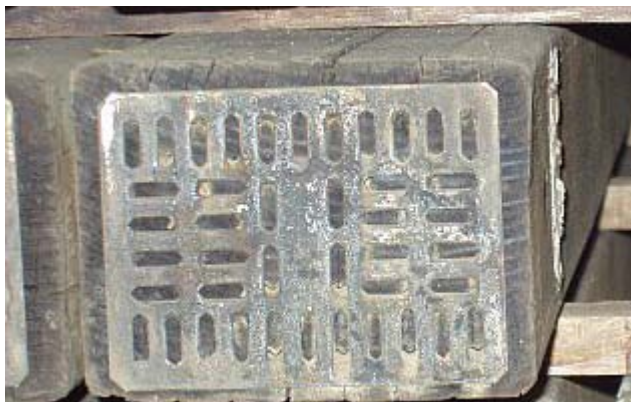
Figure III-7. Example of an end-plate on a penta treated Douglas-fir crossarm.
